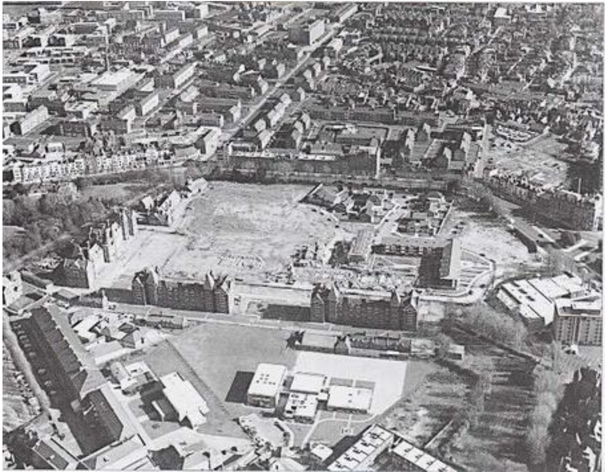
Clarence Barracks demolition. Late 1960s. Left: City Museum and City Records Office converted 1970-3
